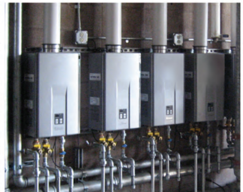
High school expands available space in mechanical room with increased efficiency and less capital expense.
